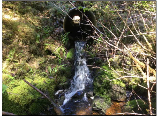
Figure 3.—Perched culvert at waypoint 107.
